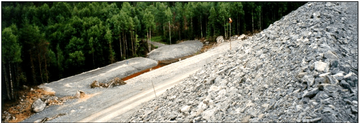
Figure 3.31: Ditch for collection and flow measuring of seepage water alongside dam [66, Base metals group, 2002]
