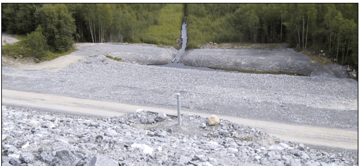
Figure 3.32: Another ditch for collection and flow measuring of seepage water alongside dam [66, Base metals group, 2002]
